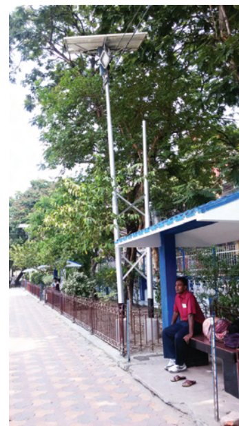
Solar Lighting at Deshapriya Park, Kolkata
