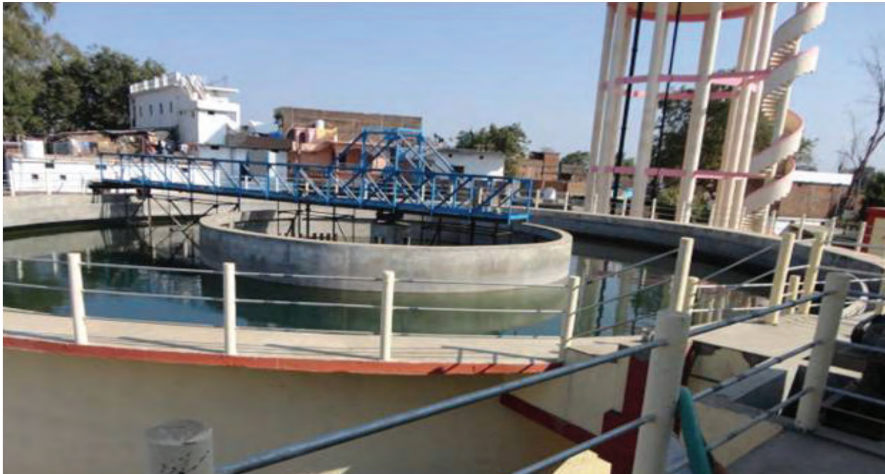
HUDCO Financed Water Supply scheme under Mukhyamantri Shahari Peyjal Yojana at Mandla, Madhya Pradesh
