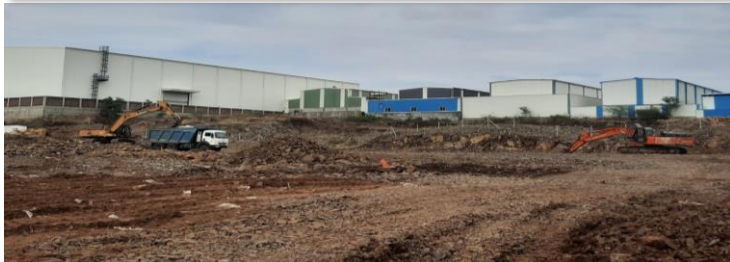
Minda Instrument Cluster Plant Pune
