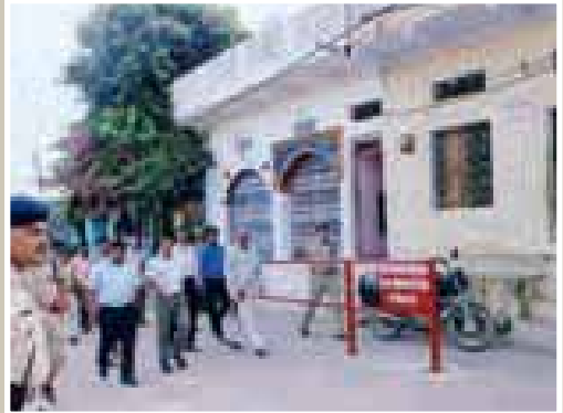
Erected iron railing in the Kamadgiri circumambulation route at renowned pilgrimage centre Chitrakoot (District : Satna) – a CSR initiative
