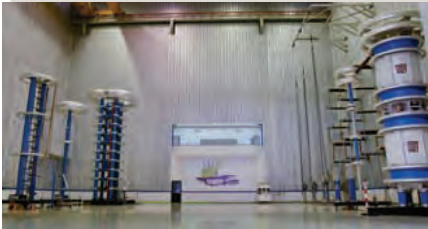
CGs newly built 550 kV EHV test laboratory at Indonesia will cater to the growing demand of EHV power transformers from electricity transmission utilities in South East Asia
