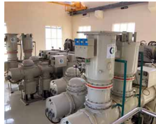
Gas Insulated Switchgears (GIS)
