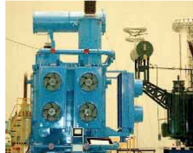
Transformers and Reactors
