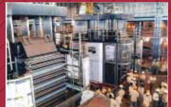
Horizontal Pressure Filters
