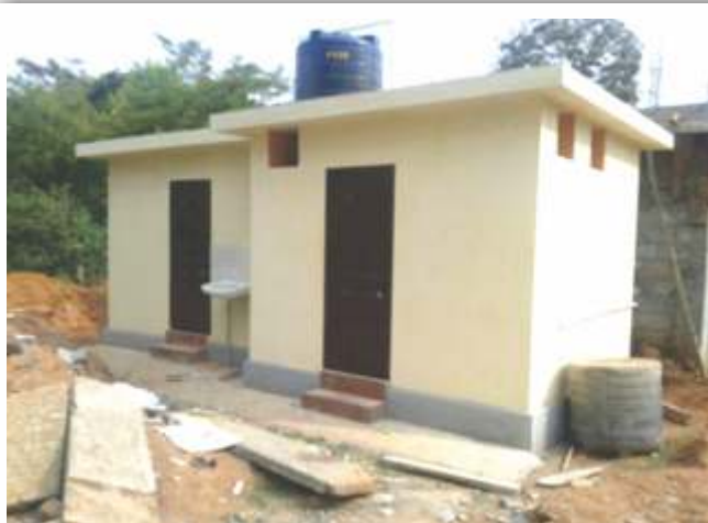
Toilets constructed under 'Swachh Bharat - Swachh Vidyalaya Abhiyan' at Government Junior College, Kalasa
