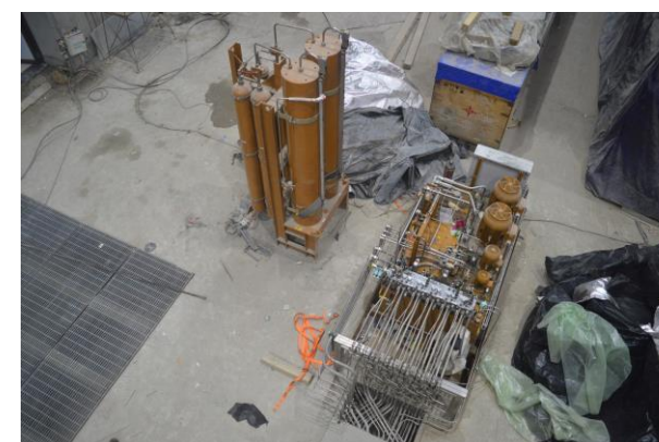
UNIT-1 HPU INSTALLED
