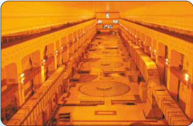
1500 MW - NJHPS (Power House)
