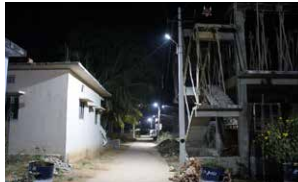
Installed 250 no.s of Energy Efficient LED street Lights to entire streets of Ankireddygudem Village in Telengana
