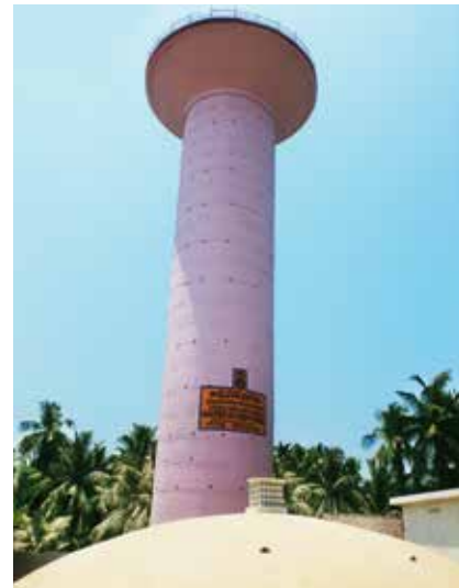
90,000 Liter Overhead Balancing Reservoir for Amalapuram Water Supply Scheme
