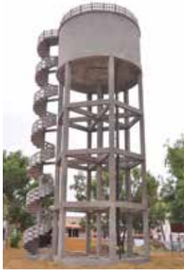
Elevated Service Reservoir of 1.3 Lakh Liter Capacity 16 Meters Staging for Palladam Water Supply Project
