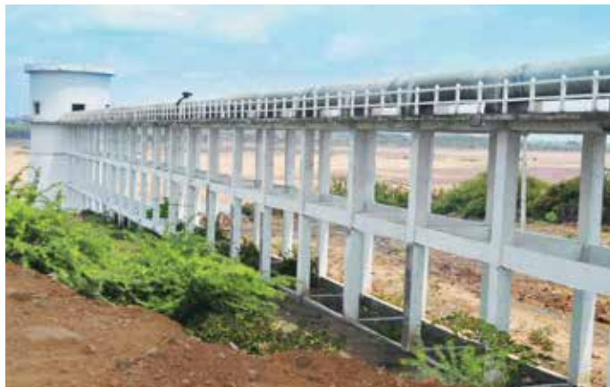
Intake Well Cum-Pump House in River Godavari for Bhadrachalam Water Supply Scheme
