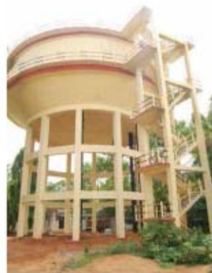
Elevated Storage Reservoir of 8 Lakh Liter Capacity
