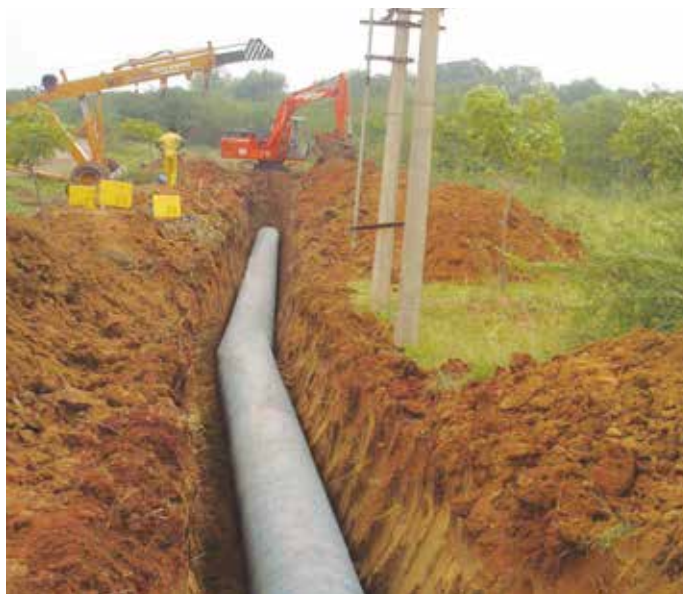
800 mm dia MS pipes for CWSS to 1751 rural habitations in Pudukottai District, Tamilnadu
