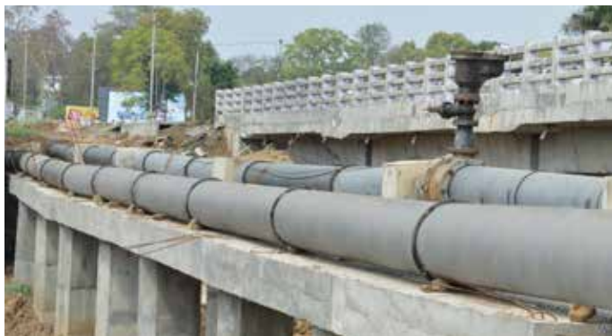
600 mm dia DI pipeline laying for Chhindwara Water supply Scheme, Madhya Pradesh
