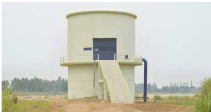
Collection well at Head Water Works at River Nagavali For Rajam Water Supply Improvement Scheme, Andhra Pradesh
