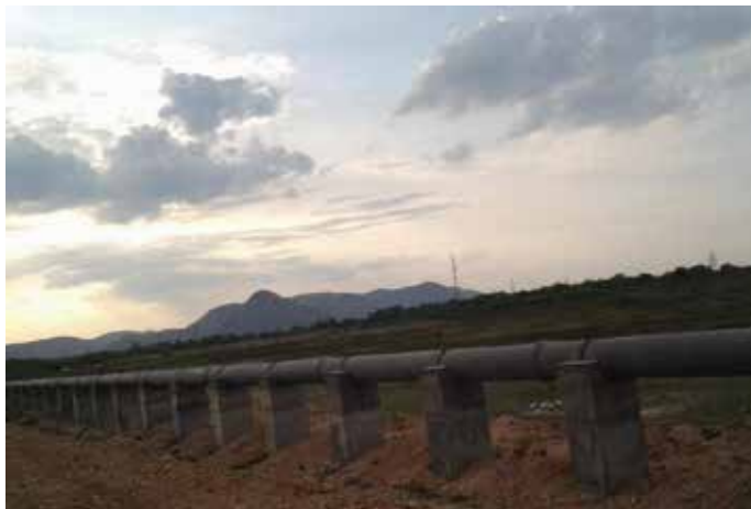
500 mm dia DI pipeline for Badvel Municipality Water Supply (Package-I), Andhra Pradesh
