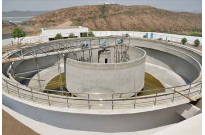
9 MLD Water Treatment Plant at Badvel Water Supply Scheme in Andhra Pradesh
