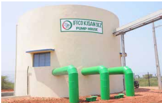
Pump House at M/s IFFCO KISAN SEZ Limited, Nellore in Andhra Pradesh
