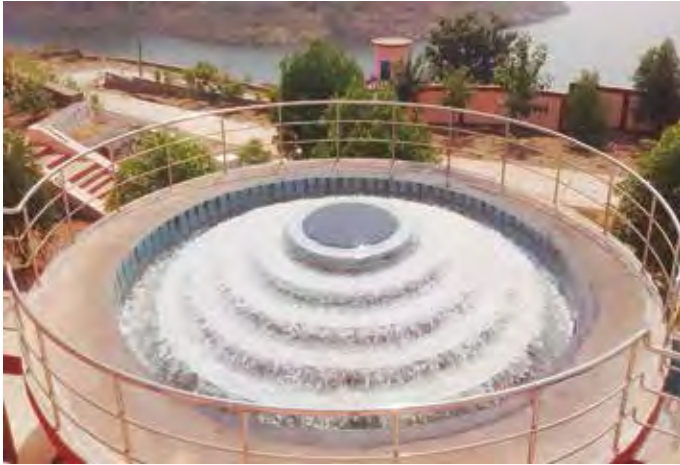
Aerator in 9 MLD WTP at Bhrammamgari Matam for Badvel Project in Andhra Pradesh
