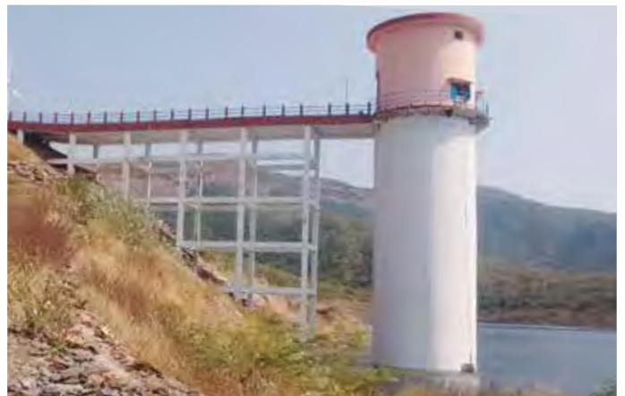
9 Mtr Dia x 30 Mtr Height Intake well at Bhrammamgari Matam for Badvel Project in Andhra Pradesh
