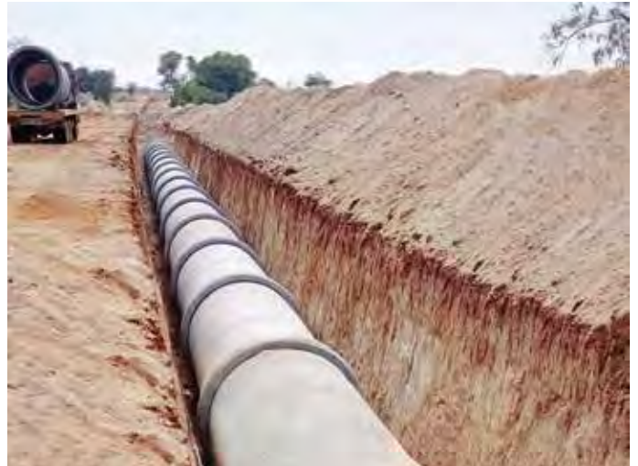
1900 mm dia PSC pipeline laying for Pulakurthy Lift Irrigation Scheme, in Andhra Pradesh
