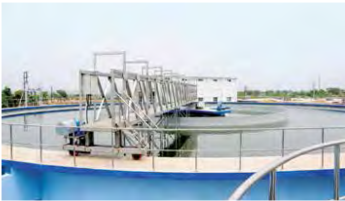
Clariflocculator in 40 MLD WTP at Indalwai for Balkonda Project in Telangana
