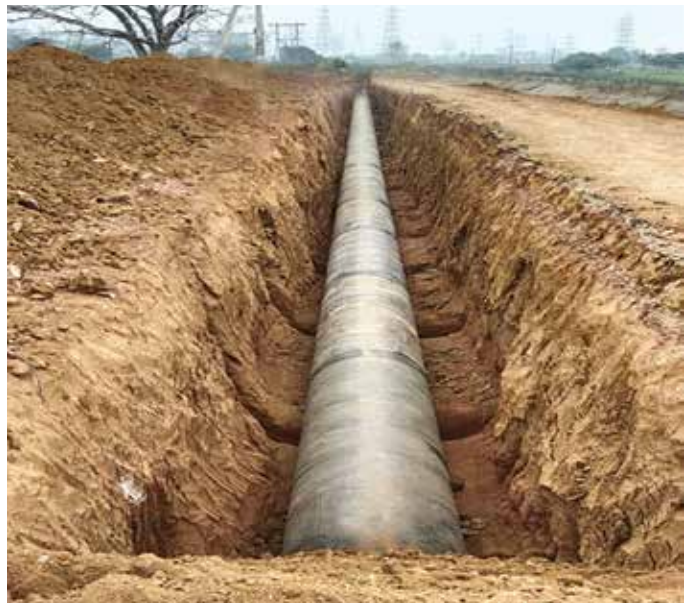
1500 mm Dia MS Pipeline laying work at Raw Water Gravity Main in Bilaspur Water Supply Scheme, in Chhattisgarh
