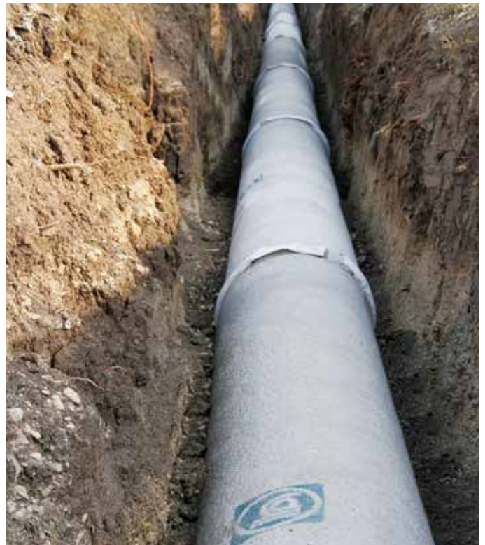
700 mm dia PCCP Gravity Main Pipeline laying at Buldhana Water Supply Scheme, in Maharashtra
