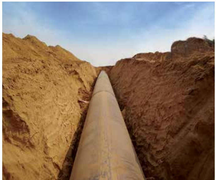
2028 mm dia outer diameter MS Pipeline laying at Tharad-Sipu Project, Palanpur Pkg-2, in Gujarat
