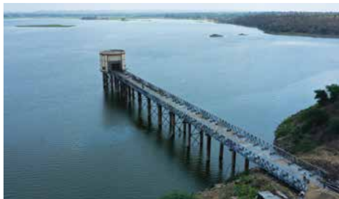
Intake well cum pump house - 13 mtr dia with Approach Bridge - 120 mtrs length x 6 mtr width based on Patadungri dam for Hafeshwar Package-6 Project, in Gujarat
