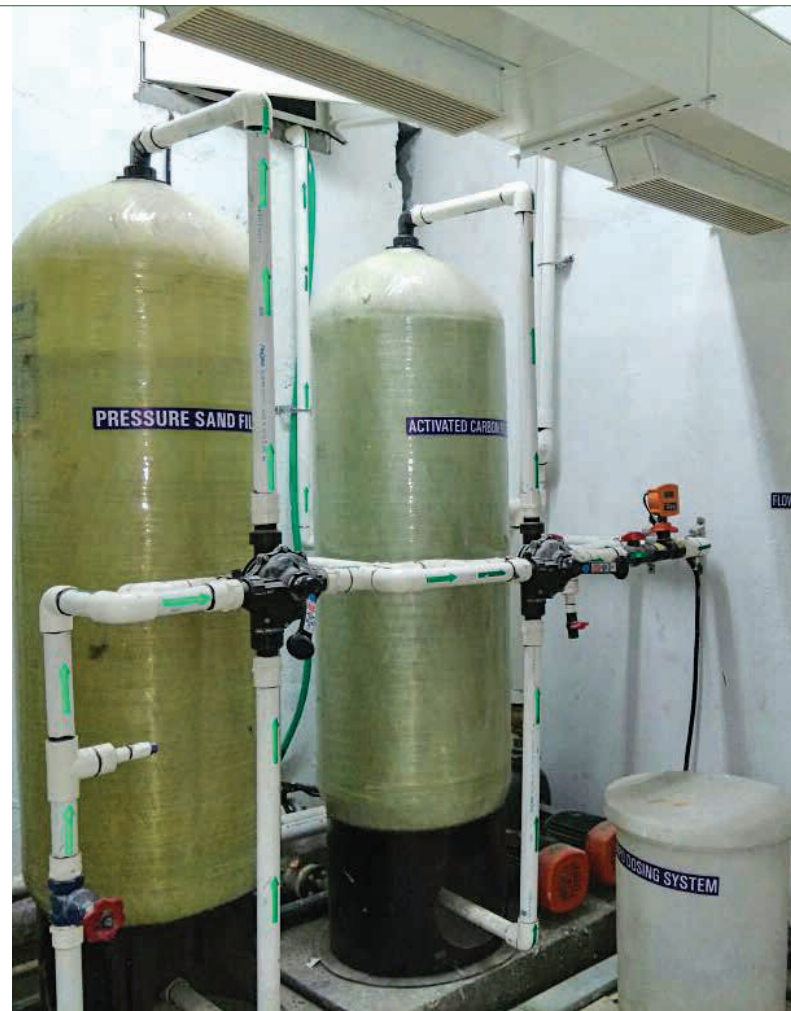
Sewage Treatment Plant
