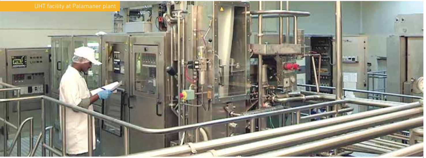
Topp Up line at Palamaner plant
