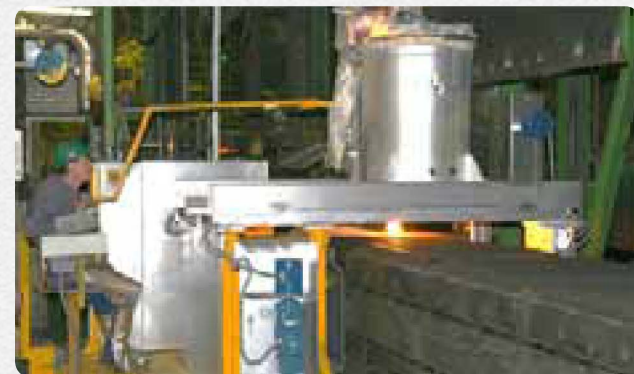
A new pouring machine for steel castings was installed into series process of the GFD moulding line at Eisenwerk Erla GmbH
