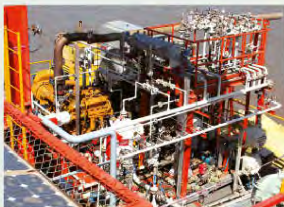
Gas Engine Driven Reciprocating Gas Compressor Package for an Unmanned Off-shore Platform
