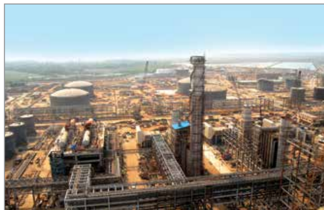
366 MW CCPP at IOCL's Paradeep Refinery
