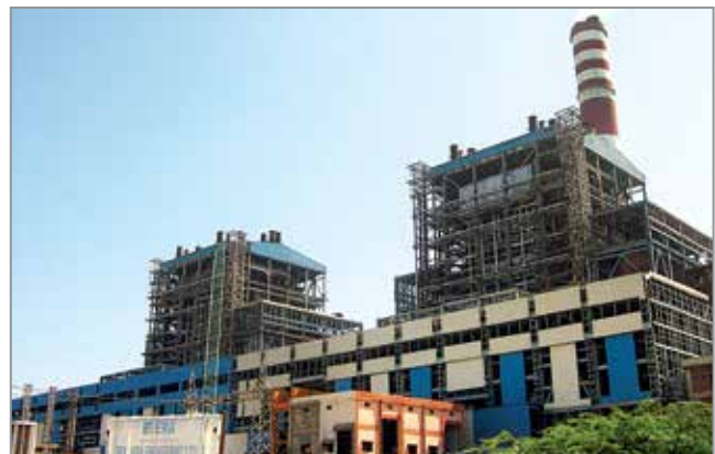
2x600 MW North Chennai TPS-commissioned India's first indigenously manufactured sub-critical set of 600 MW on EPC basis
