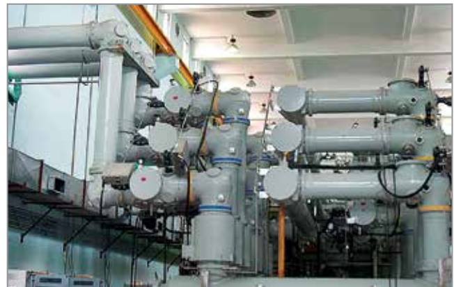
400 kV GIS commissioned for 2x600 MW North Chennai TPS Stg-II, Unit-2
