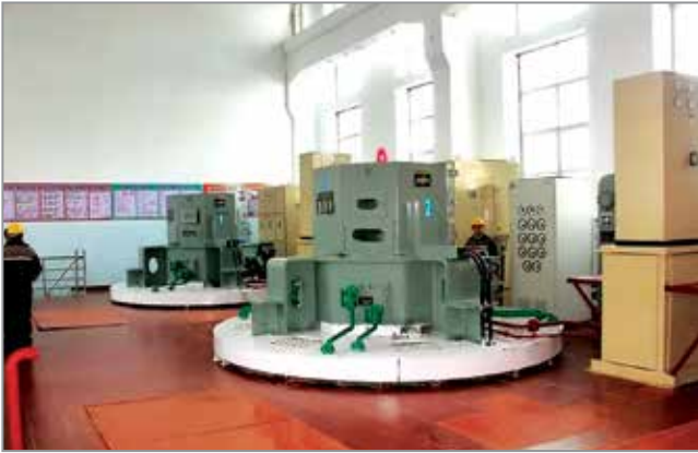
2x4.75 MW Modernisation & Uprating of Varzob Power Plant commissioned and project handed over to Govt. of Tajikistan
