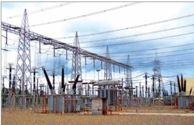
400 kV Substation at Gas-based Power Plant, OTPC-Palatana
