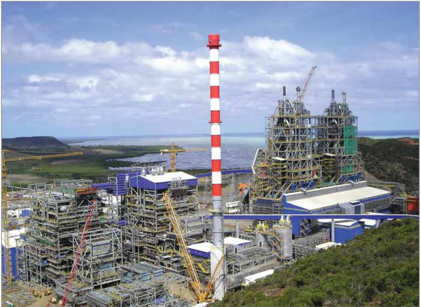
Two nos. 135 MW Circulating Fluidised Bed Combustion (CFBC) Boilers under commissioning at New Caledonia
