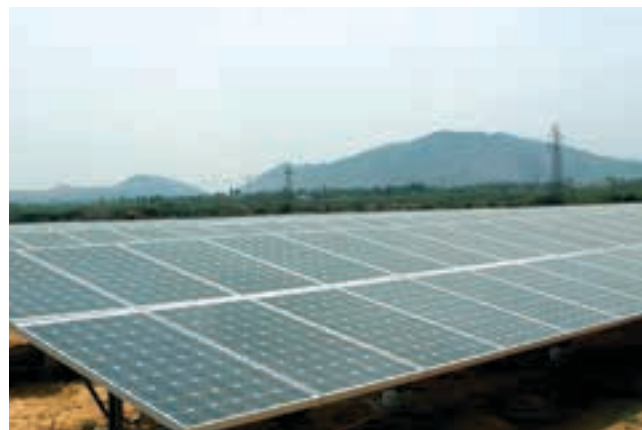
Grid Interactive Solar Power Plant of 5 MWp capacity installed at BAP Ranipet as part of Energy Management initiatives across BHEL
