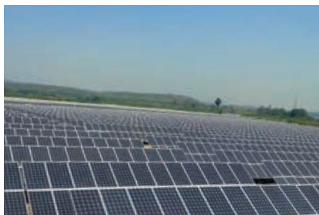
10 MW Solar Power Plant commissioned at NTPC Talcher
