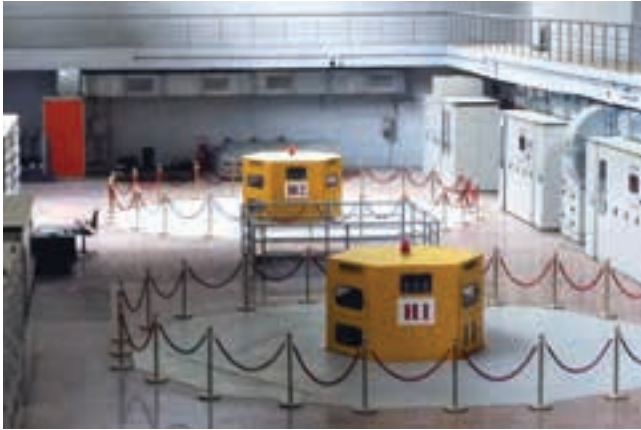
2x100 MW Unit 2 of Nam Chien Hydro Project executed in Vietnam
