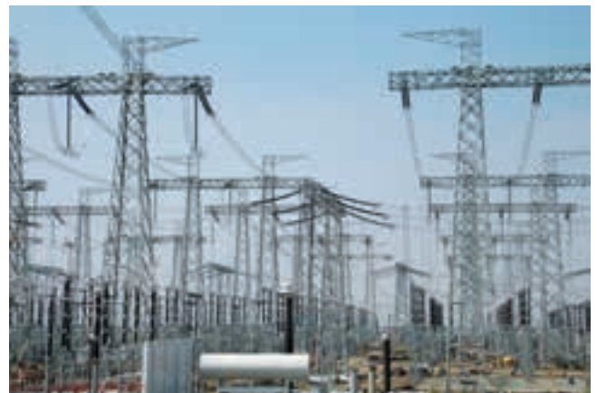
Constructed and successfully commissioned 765/400 kV substation 6 months ahead of schedule at Raichur in Karnataka
