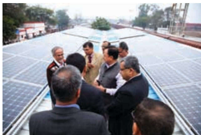
25 kW Roof-top Solar Power Plant using platform shelter at Gurgaon Railway Station commissioned for RITES
