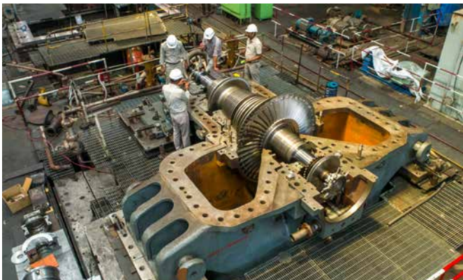
150 MW steam turbine for captive power plant at BHEL works at Hyderabad
