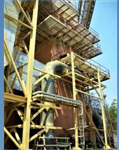
Seawater FGD system for Trombay 1x250 MW
