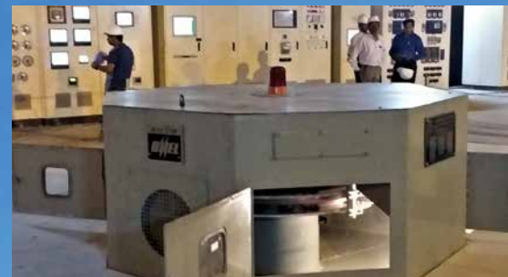
Turbine Hall of 4x180 MW Mangdechhu HEP project
