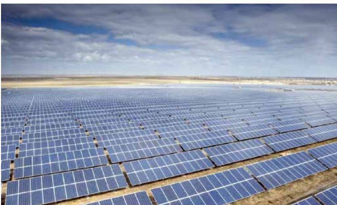
65 MW Gujarat Solar Park near Charanka village, Gujarat. BHEL has commissioned 15 MW capacity on EPC basis.
