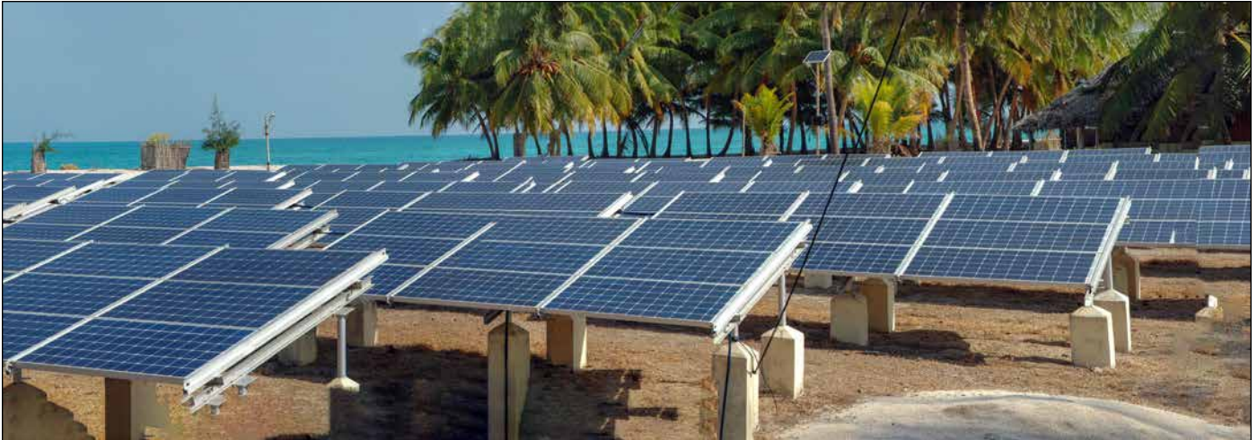
BHEL has commissioned solar photovoltaic power plants of cumulative capacity of over 2 MW at various islands in Lakshadweep
