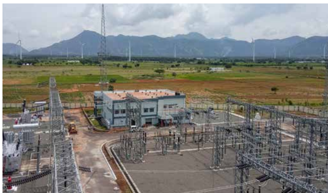
Thappkundu Substation (400kV - 9 bays, 110 kV - 12 bays) for TANTRANSCO commissioned by BHEL in October 2018
