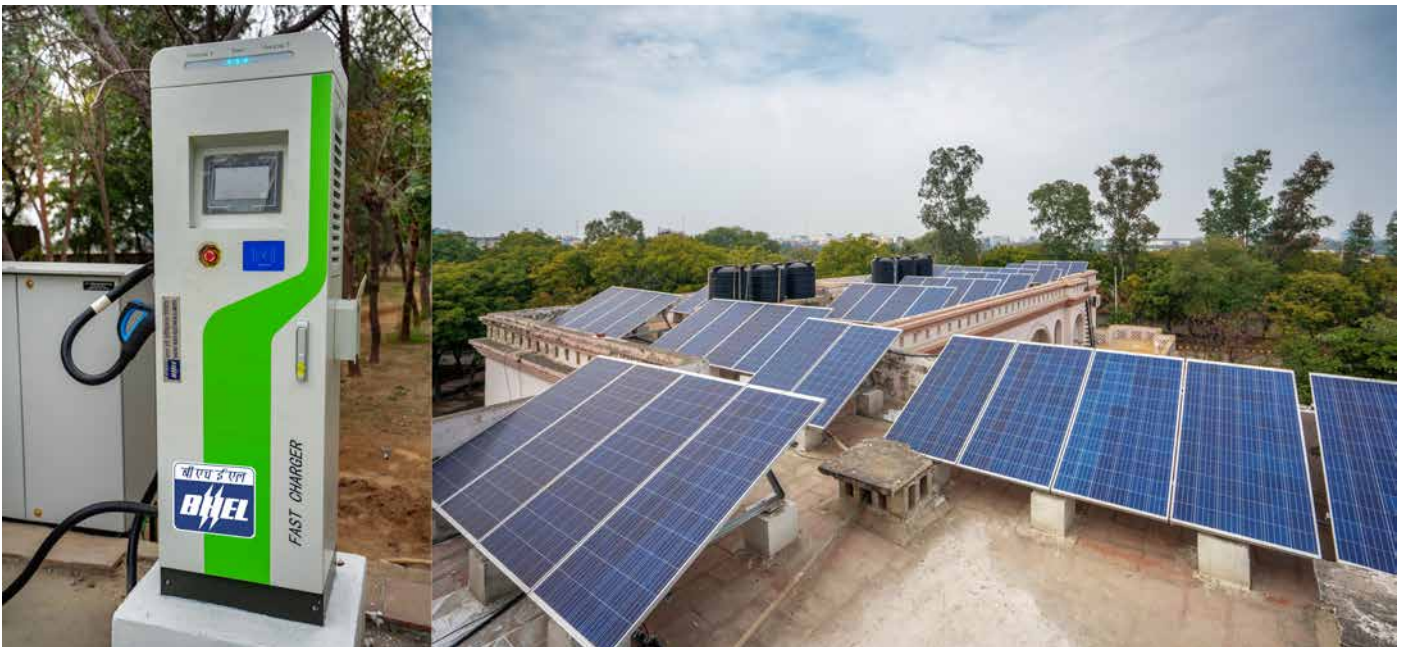
Solar PV based electric vehicle charging stations commissioned along Delhi-Chandigarh highway
