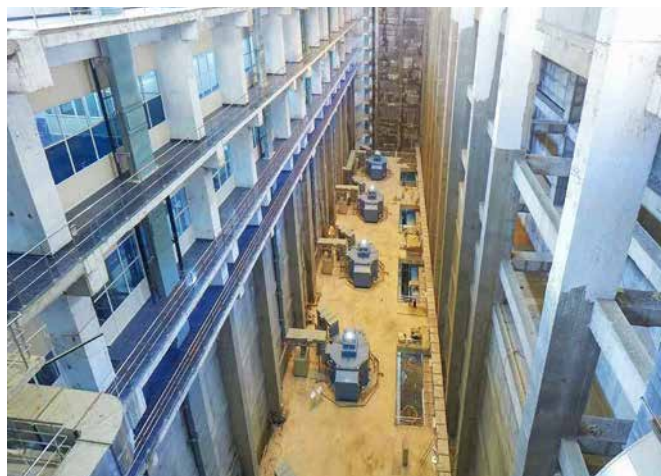
Turbine Hall of BHEL commissioned 5x30 MW Kalwakurthy Lift Irrigation Scheme (LIS)
