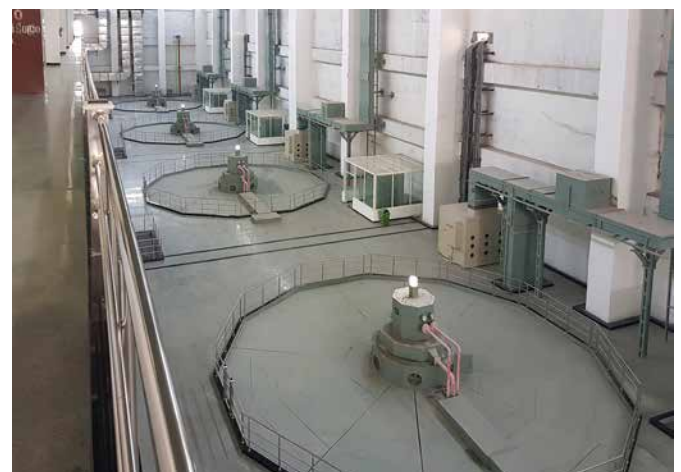
Bay hall of 4X30 MW Pullichintala hydroelectric project in Telangana, commissioned by BHEL
