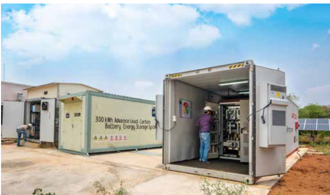
1 MWh grid-connected Battery based energy storage system (BESS) designed and developed by BHEL, installed at Corp R&D, Hyderabad
