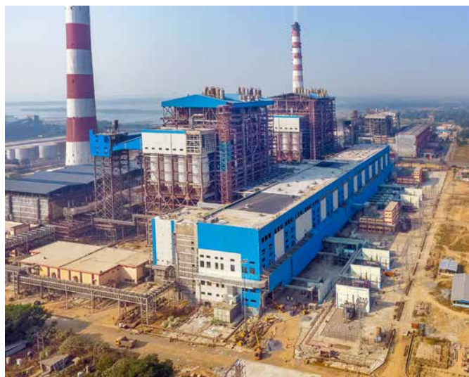
Both supercritical units of 2x660 MW Ib Valley project were synchronised in 2018-19 and made ready for capacity addition by BHEL
