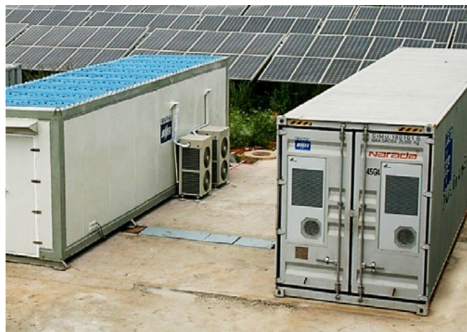
BHEL is executing its maiden order of setting up of a cumulative 410 kWh Battery Energy Storage Systems (BESS) for TERI
