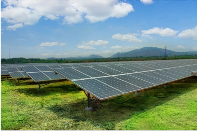
5MW in-house Solar PV installation at BAP, Ranipet for captive power generation
