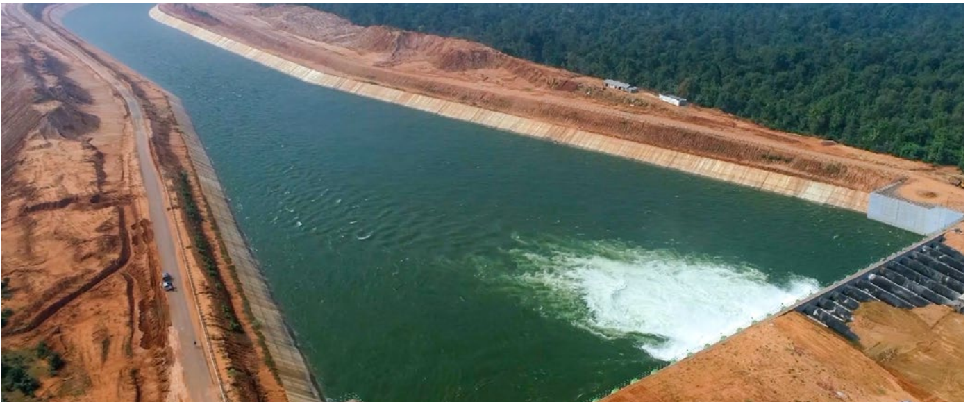
BHEL has commissioned the pumping units for Kaleshwaram Lift Irrigation Scheme, Telangana - world's largest LIS project
