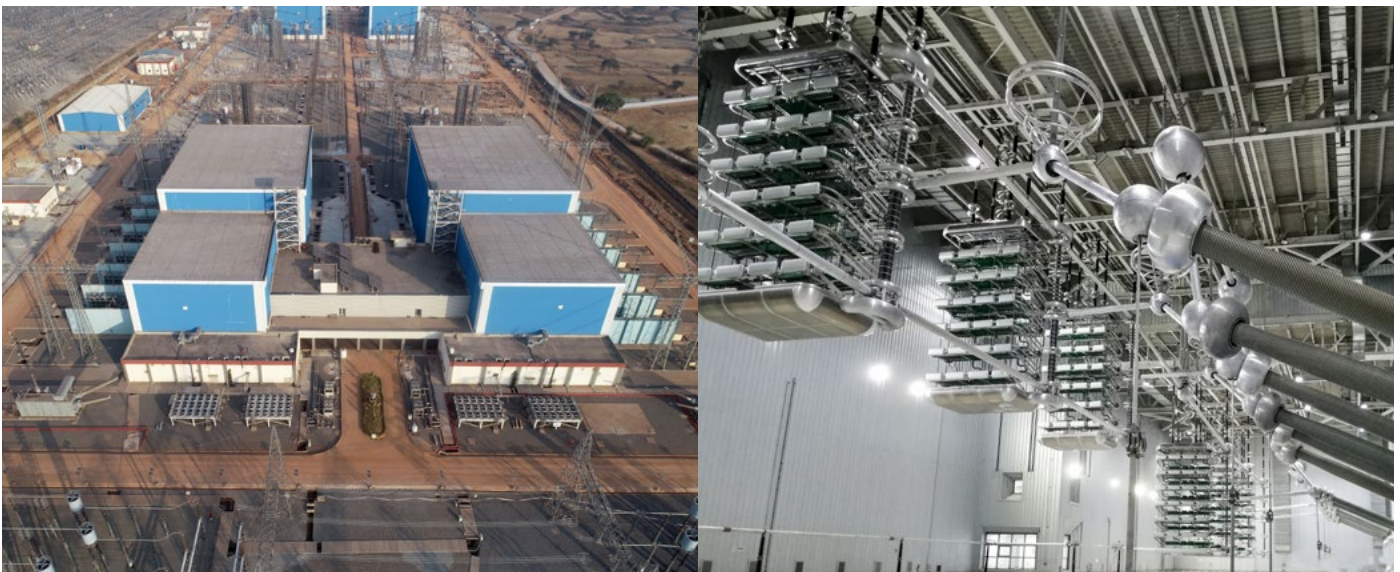
Aerial view and HVDC hall of Raigarh substation of the ± 800 kV, 6000 MW Raigarh-Pugalur HVDC link commissioned by BHEL
