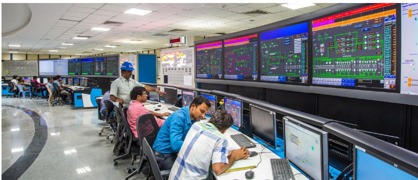
State-of-the-art control centres for power plant operations have been set up at all its commissioned units by BHEL
