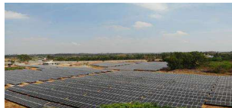
Solar Panels at HRGRDC, Bengaluru
