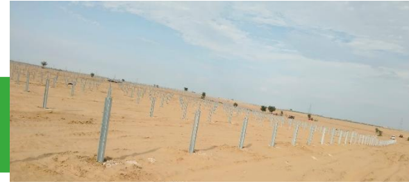
450 MWp Ground Mounted project at Bikaner, Rajasthan
