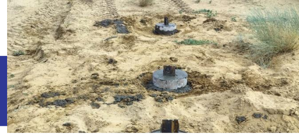
435 MWp Ground Mounted project at Bikaner, Rajasthan
