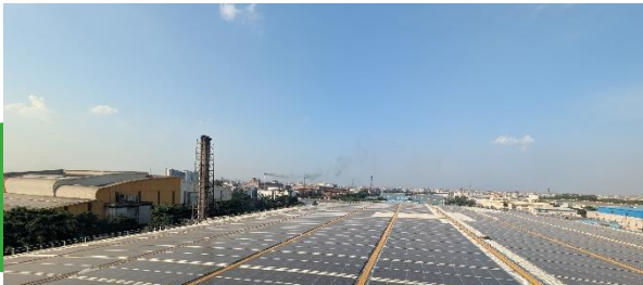
1.7 MWp Rooftop project at Noida, Uttar Pradesh
