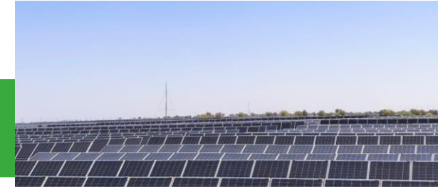
412.5 MWp Ground Mounted project at Bikaner, Rajasthan
