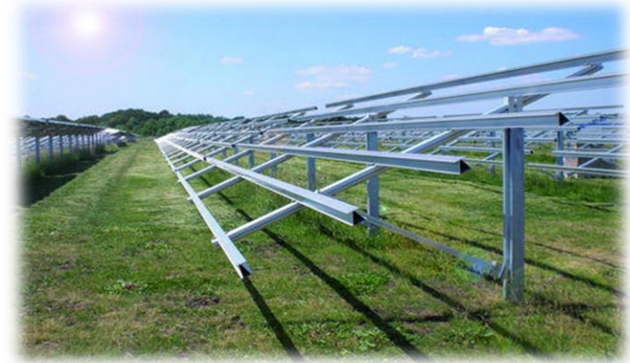
Solar Module Mounting Structures/Panels
