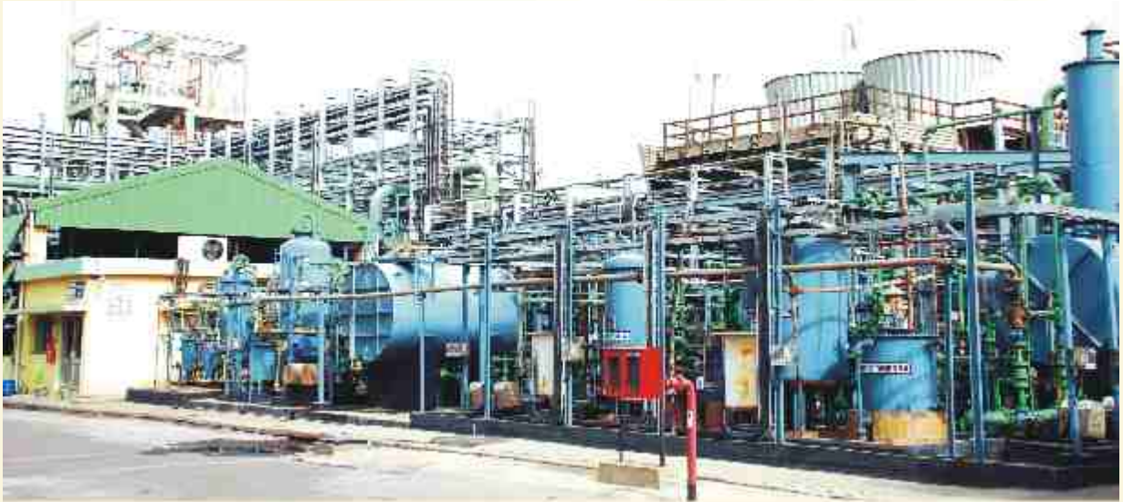
DM Plant at Membrane cell block, Renukoot
