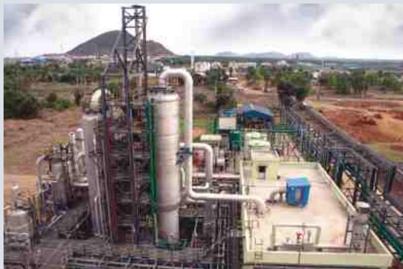
Formaldehyde Plant, Vishakhapatnam
