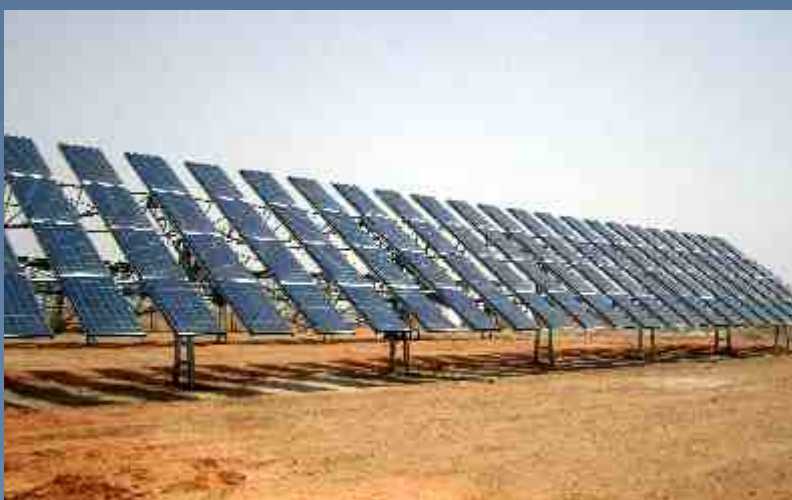
Solar Energy Panels, Phalodi, District Jodhpur, Rajasthan
