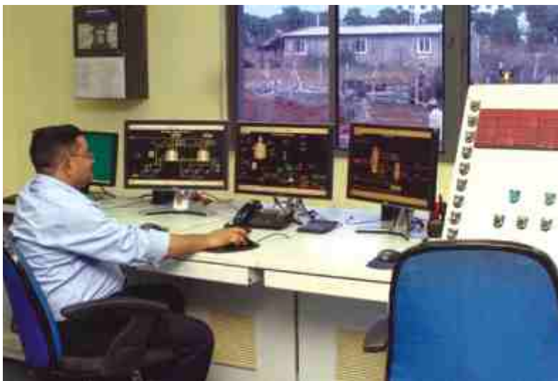
Control Room, Vishakhapatnam
