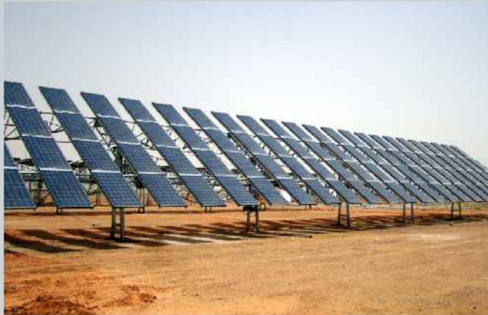
Solar Energy Panels, District Jodhpur, Rajasthan
