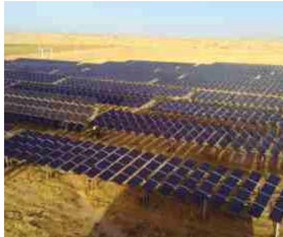
Solar project, Village Bap, District Jodhpur, Rajasthan
