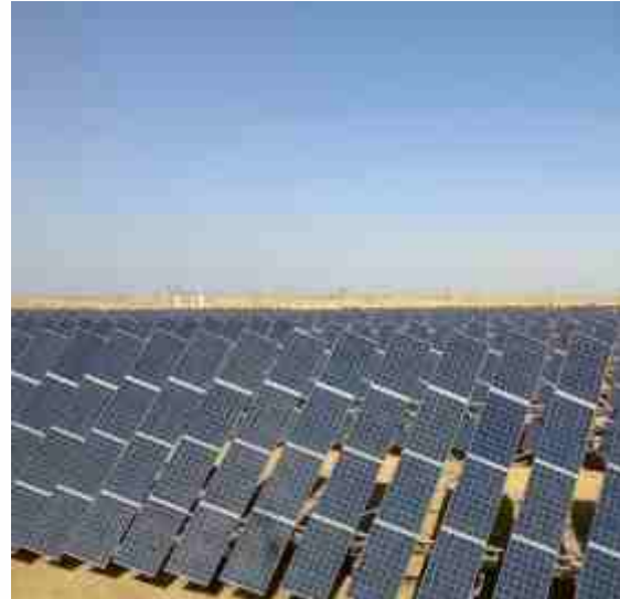
Solar Project, Village Bap, District Jodhpur, Rajasthan
