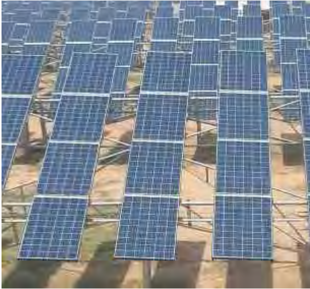
Solar Panels, Jodhpur
