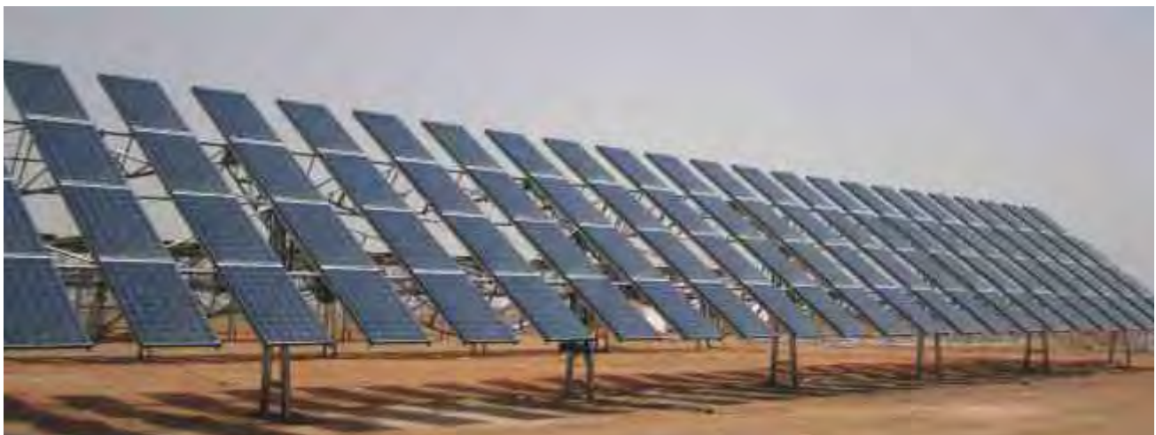
Solar Panels, Jodhpur
