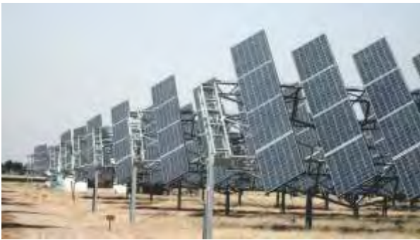
Solar Panels, Jodhpur
