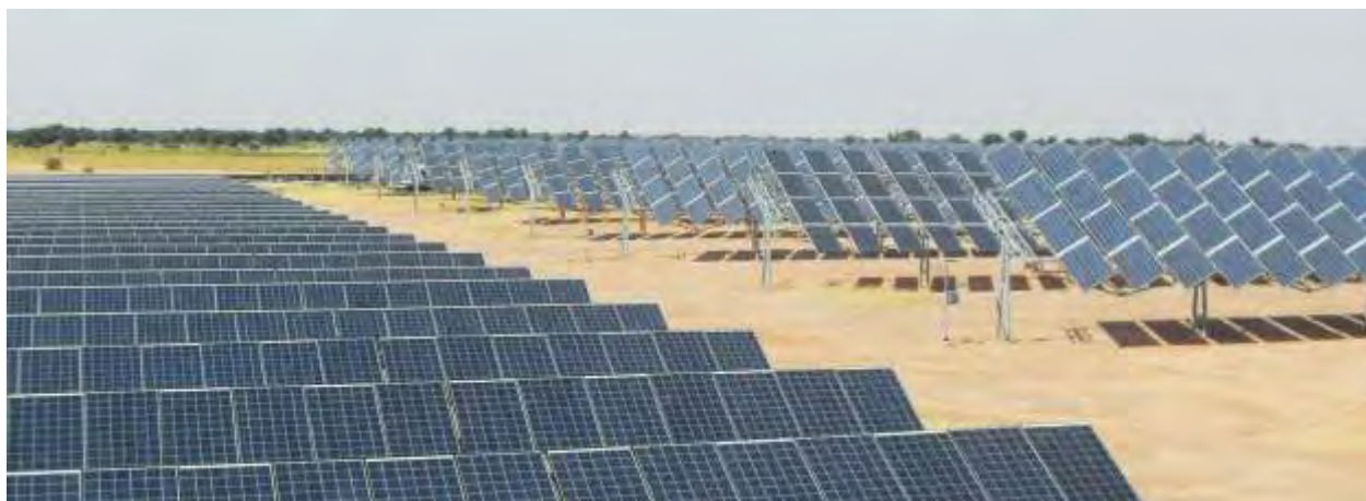
Solar Panels, Jodhpur
