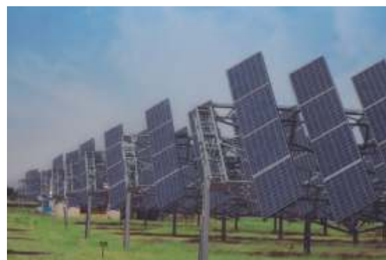
Solar Panels, Bap-Rajasthan
