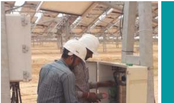
Control Panels, Solar Plant, Bap-Rajasthan
