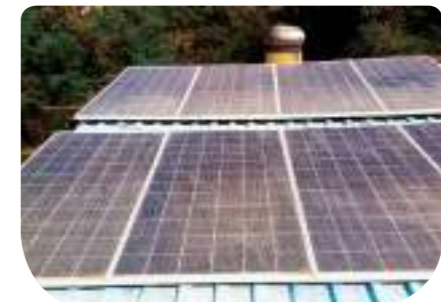
Solar Setup for school in remote area, Vasind, Maharashtra
